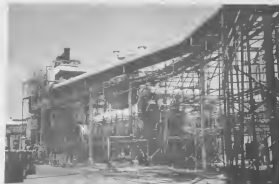
PRESENTLY Under repair is the exit gas line from SAK plant to Acid Plant that carries sulphur dioxide and other noxious materials to the disposal faraway.
